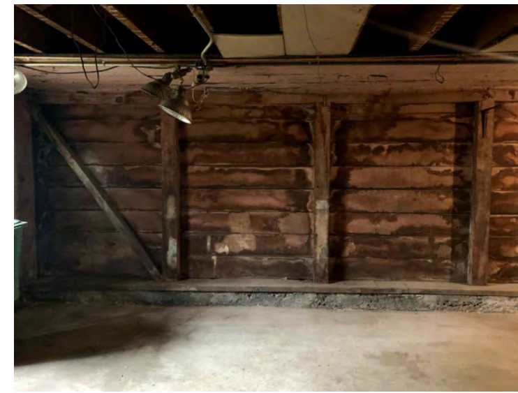
INTERIOR VIEW OF WATER DAMAGED SOUTH PROPERTY LINE WALL INSIDE (E) GARAGE
